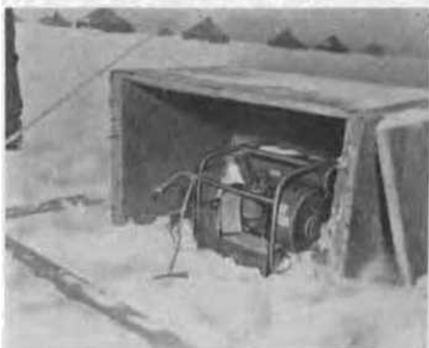
Figure 226. PE-214 in snow shed.
