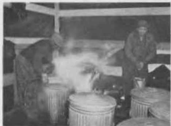
Figure 201. Interior view of snow melting plant.
